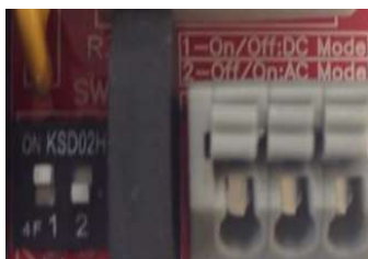
For AC Mode, #1 switch turn "ON" and #2 switch turn "OFF"
